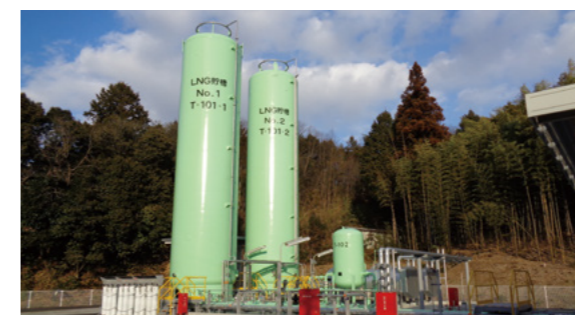
LNG fueling station set up in the Sho-o Hub Industrial Park
