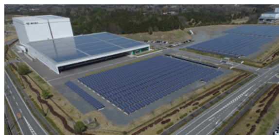
Photovoltaic power generation facilities in the West Japan Distribution Center
